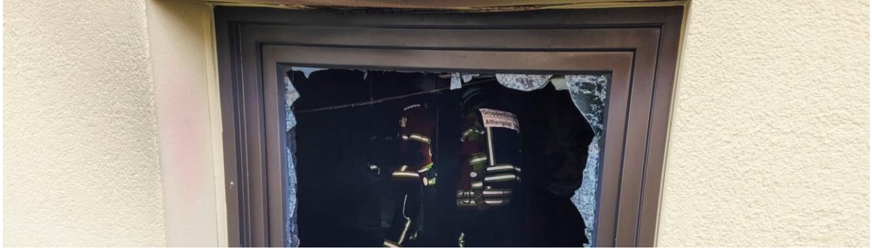
Figure 15 – Window damaged by explosion [23].
