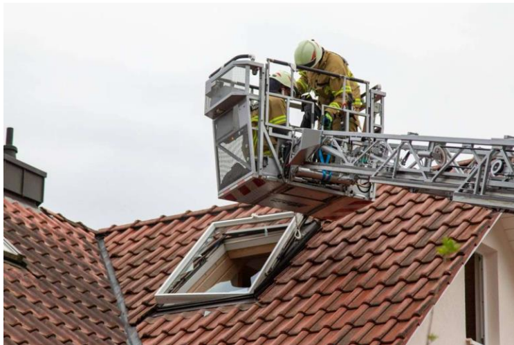
Figure 9 – Damage to window during incident [16].
