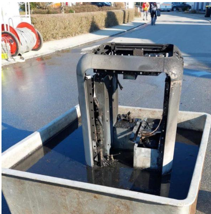
Figure 11 – ESS unit condition after firefighting operations [11].
